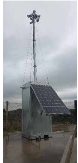
Single Solar Panel on Tower
